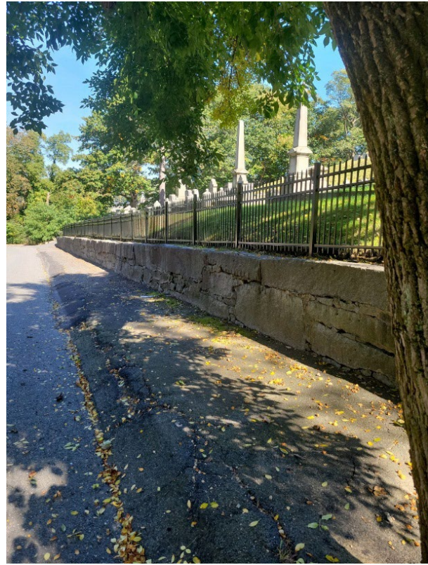
Laurel Hill Fence repair-mower damage
